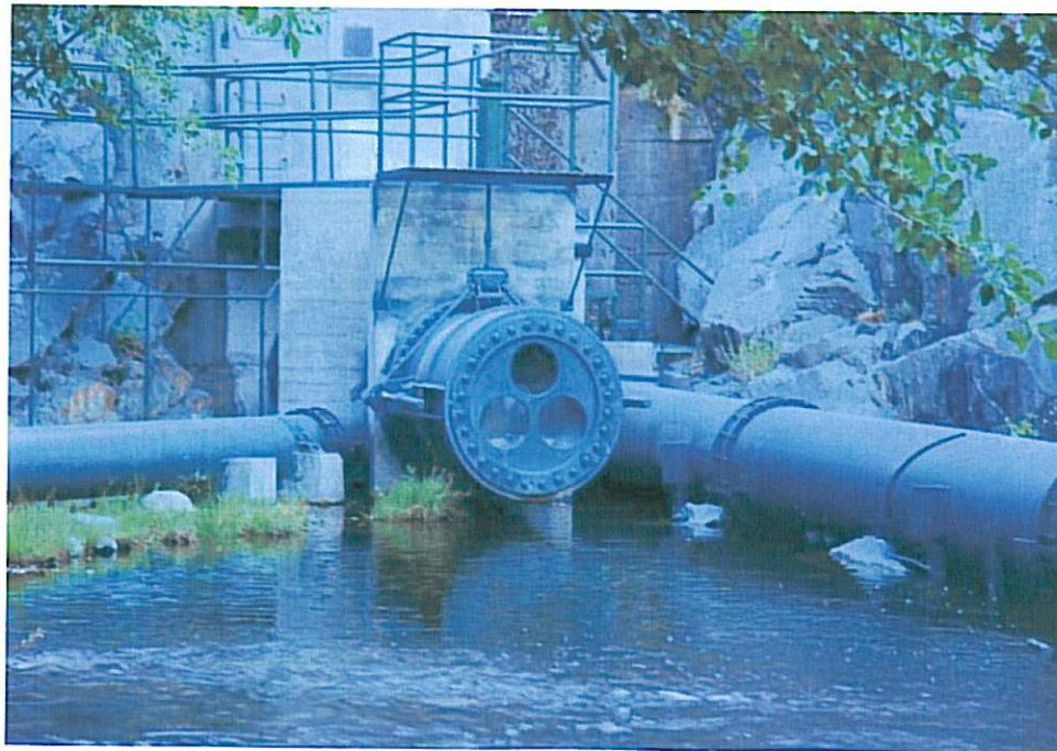
Dam Low Level Discharge Ring Jet Valve
