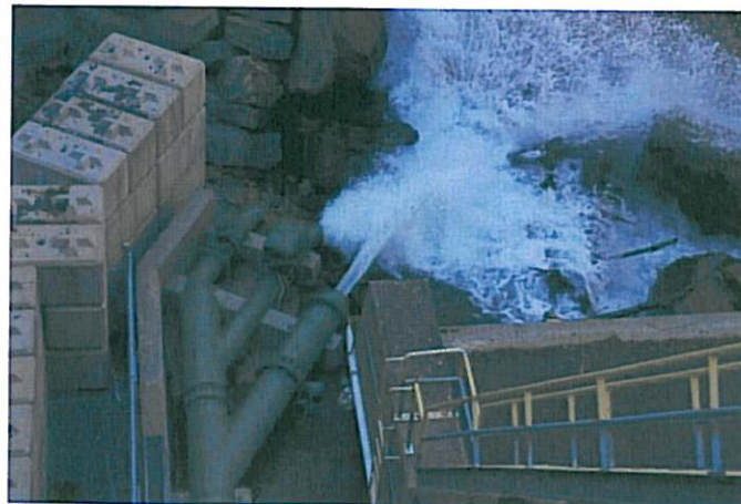
Instream Flow Pipes
