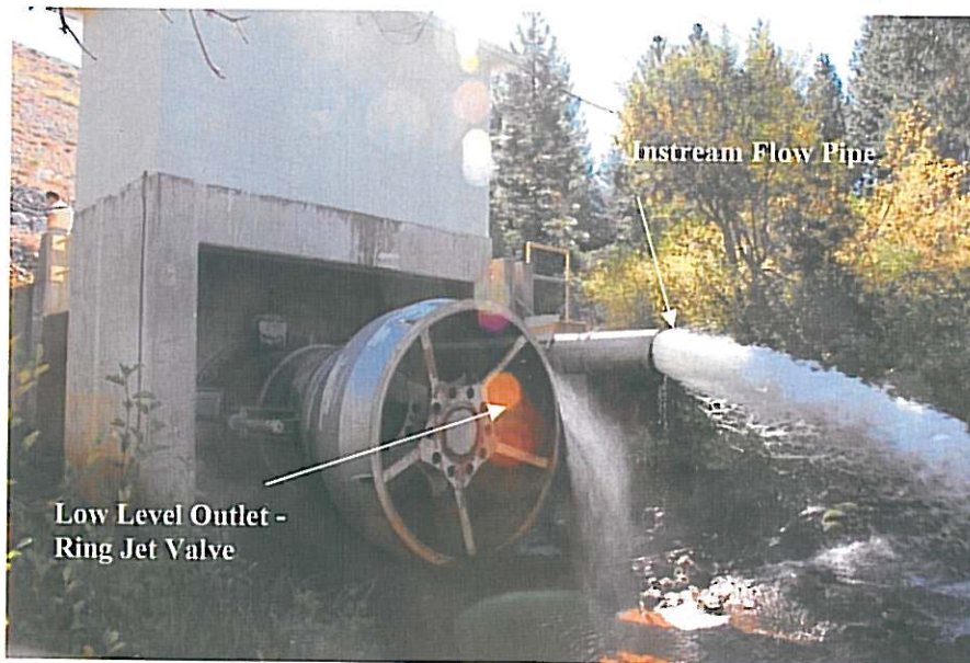
French Meadows Outlet Works - Instream Flow Pipe and Low Level Outlet
